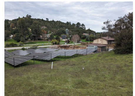
⑥ View of solar array to the northwest.
