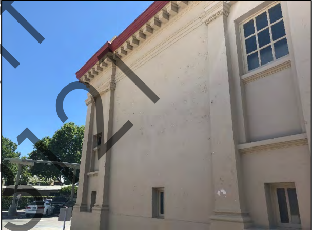
Peeling paint and stucco/plaster throughout
