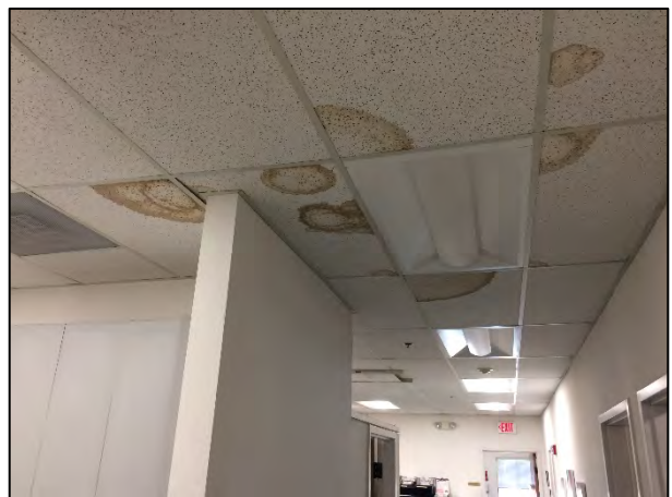
Stained ceiling tiles
