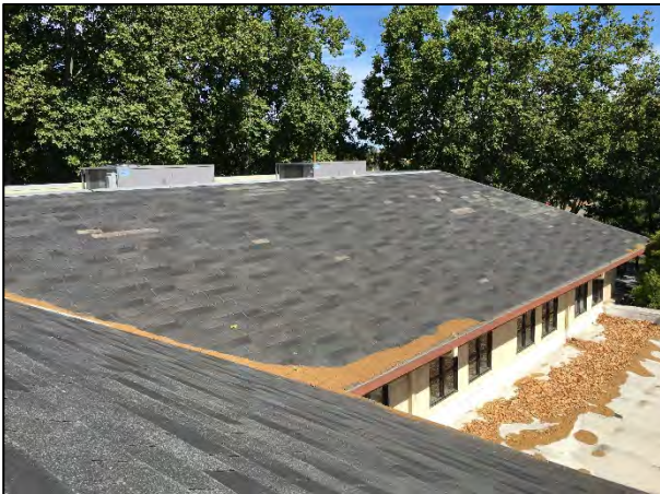
Failing Asphalt Shingle Roof
