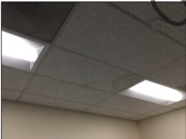
Water stained ceiling tiles
