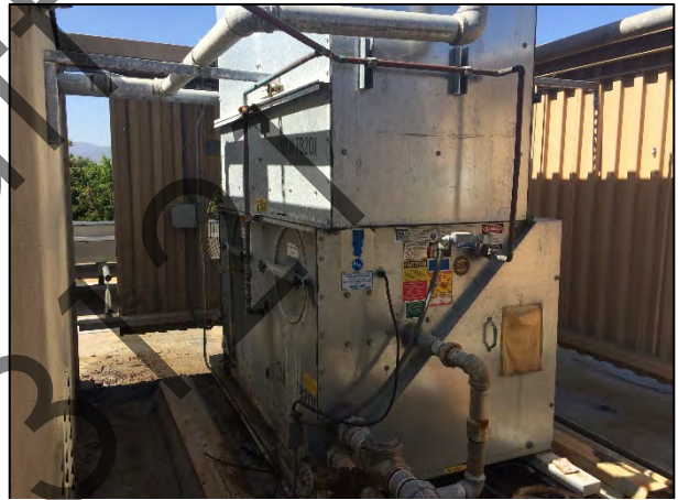
Roof top HVAC unit
