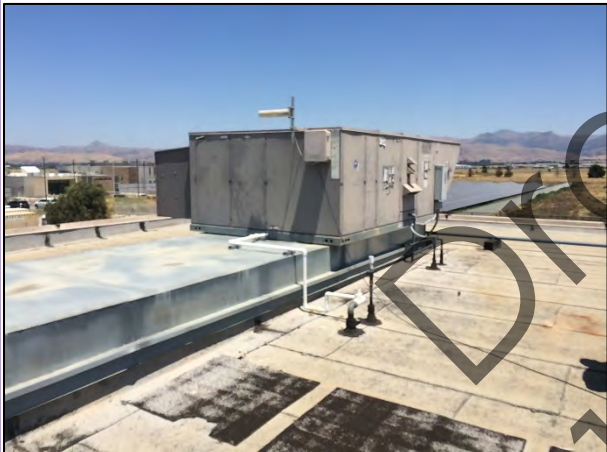
Roof Top Unit at end of useful life
