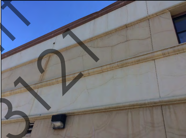
Stucco badly stained and cracked
