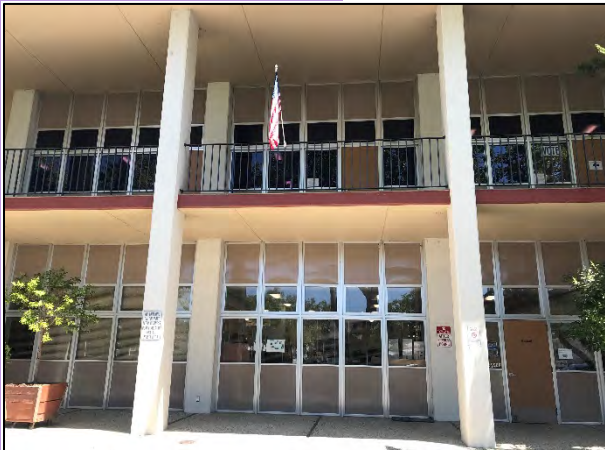
Exterior showing uninsulated curtainwall
