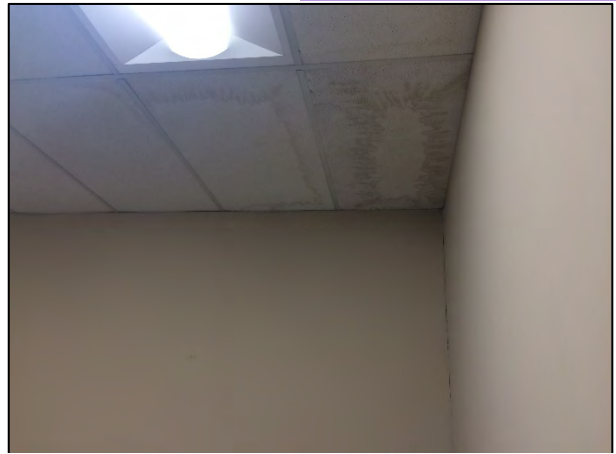
Stained ceiling tiles
