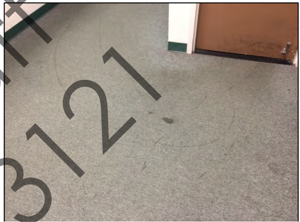
Badly stained and worn carpet
