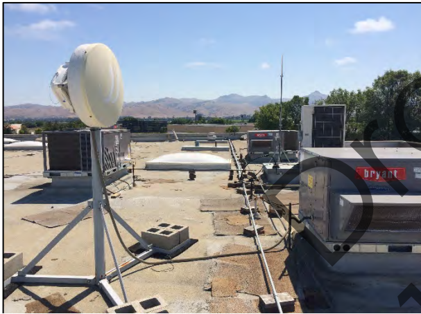
New equipment, old roof
