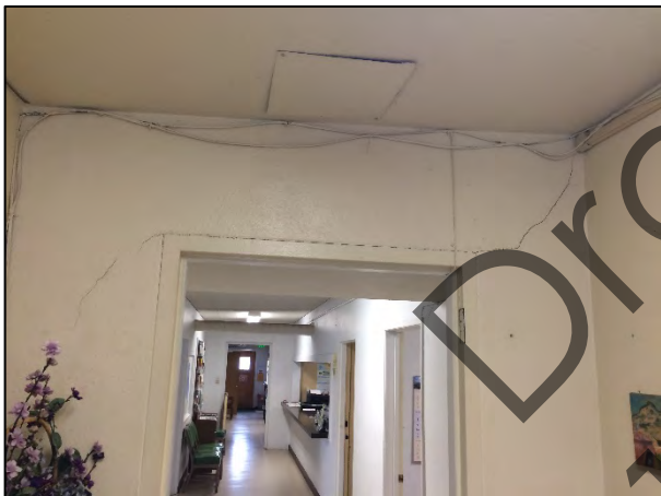
Hallway with exposed wires and wall cracks
