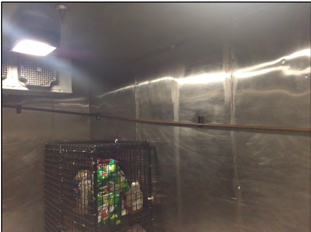
Walk-in Box panels rusting from condensation
