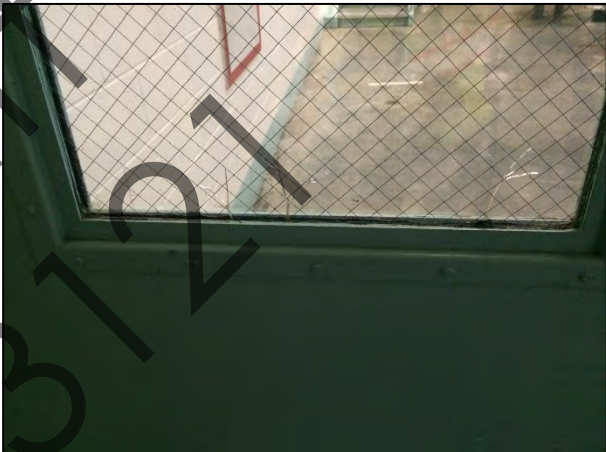
Cracks in security glazing
