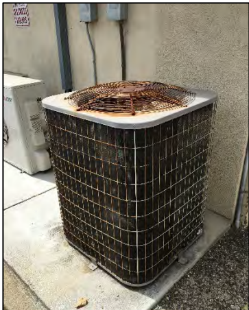
Cooling Condensing Unit
