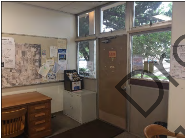
Outdated exterior wall system
