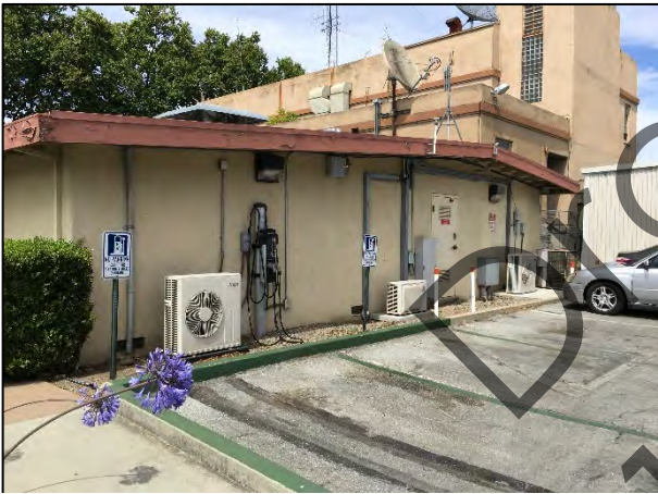
View showing cooling for NOC1 and Server
