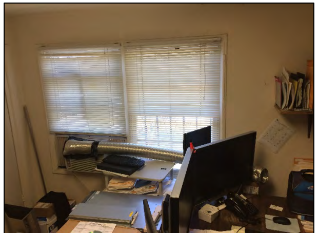
Office with window air conditioner and duct
