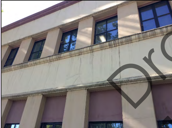
Stucco badly stained and cracked
