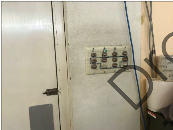
Outdated lighting controls
