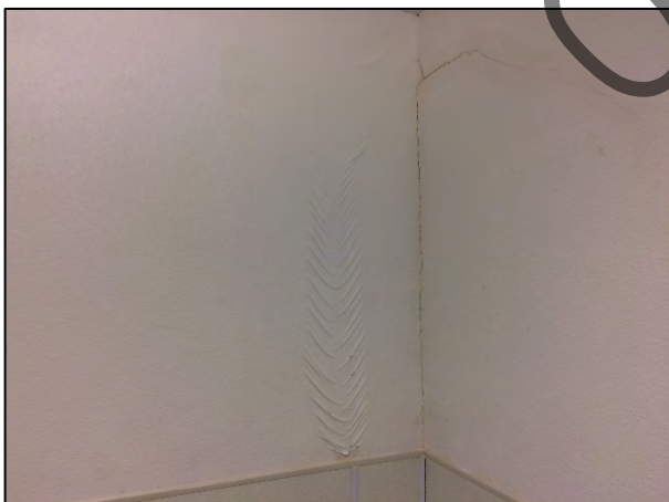
Water damage in restroom
