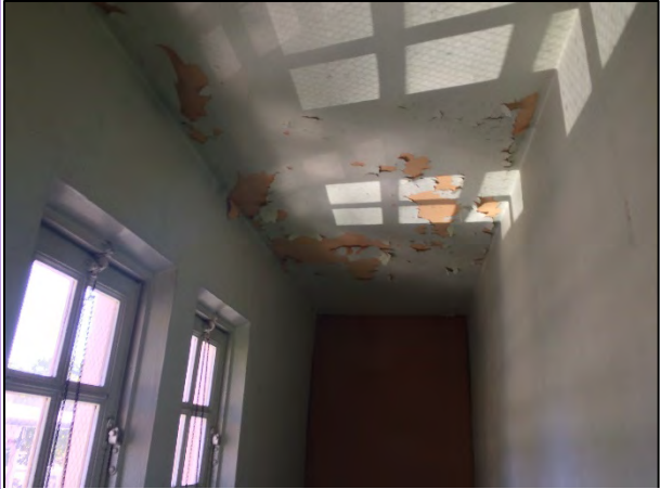
Peeling paint at ceiling
