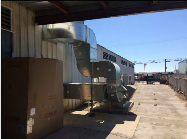
New HVAC Unit for Phase 2
