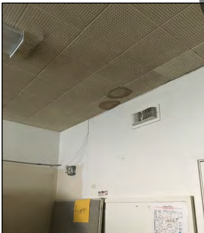
Interior water damage
