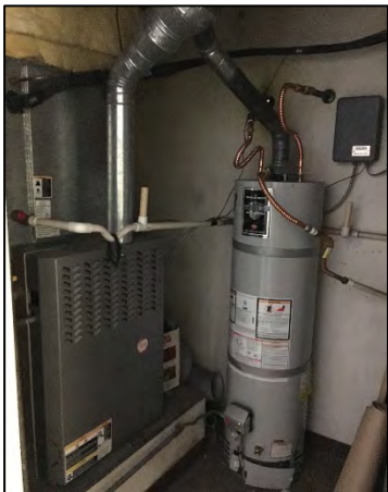
Water heater & furnace
