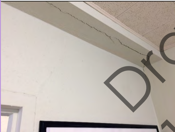
Cracking at wall/ceiling
