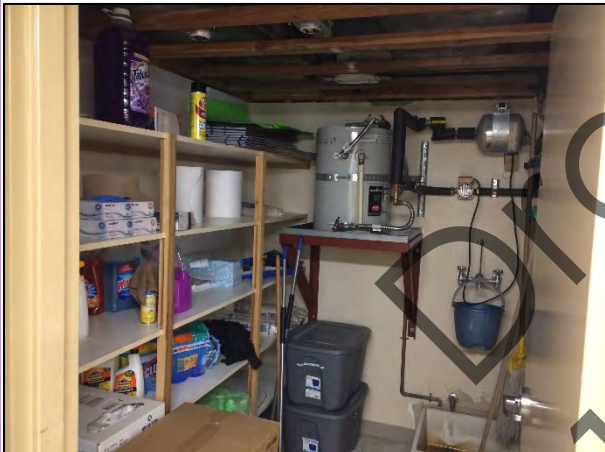
Janitor Closet with Water Heater
