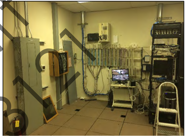
Server Room with raised floor
