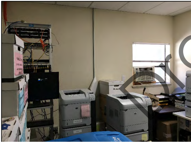
Server Room with Window A/C
