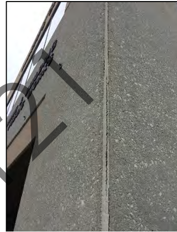
Failed joint sealant, typical
