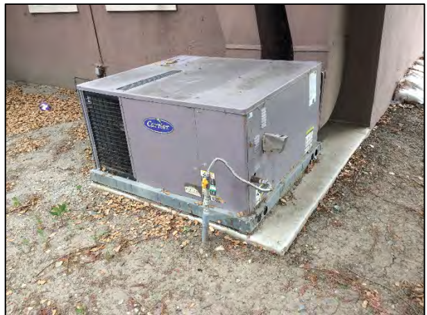
Ground Mounted HVAC Unit
