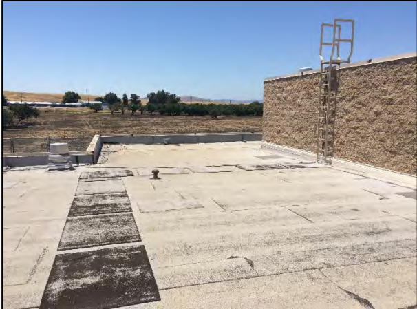
Roof at end of useful life
