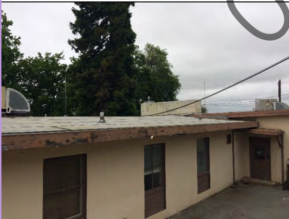
Failing Low Slope Roof
