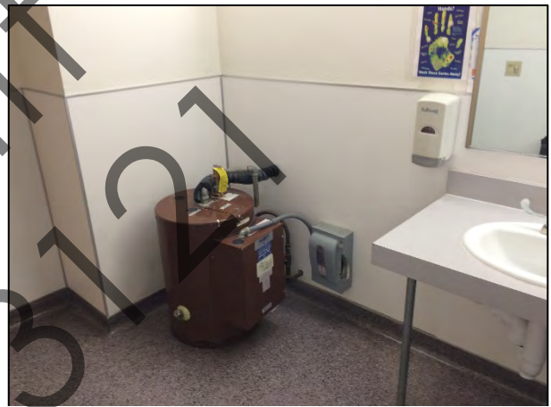
Restroom with water heater
