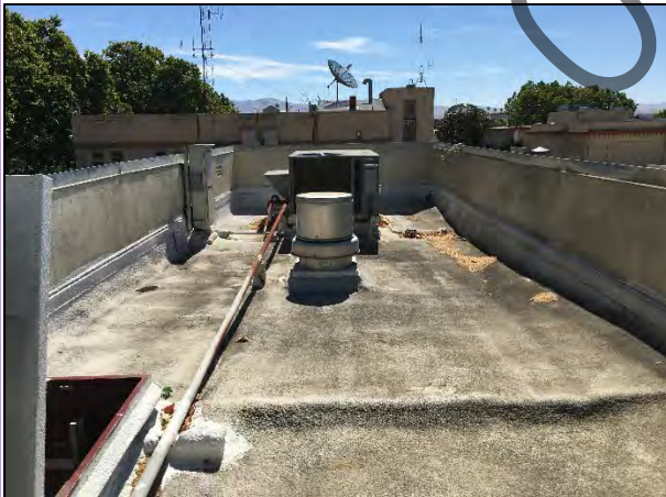
Failing Low Slope Roof
