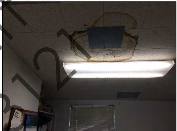
Stained ceiling tiles from roof leaks
