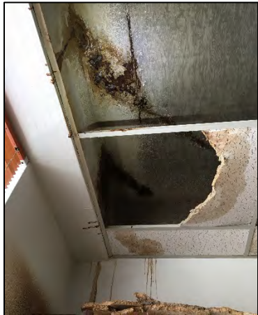
Water damage in structure
