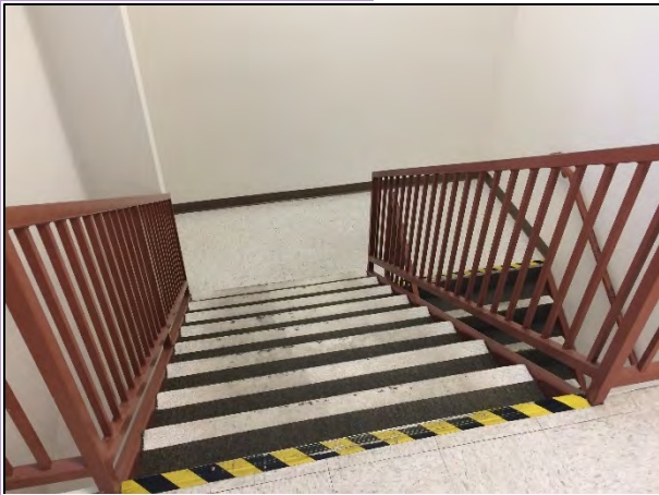
Stair with non-compliant handrail
