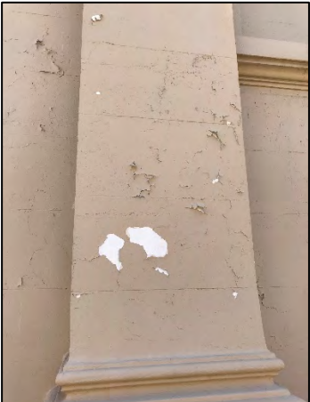
Closeup of peeling
