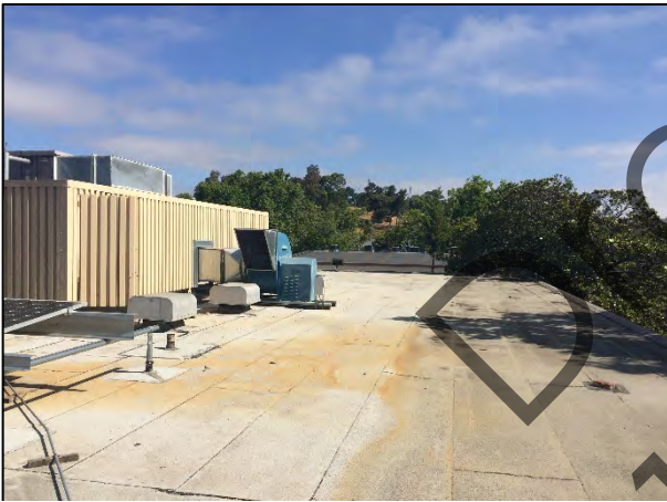
Roof with stains from standing water
