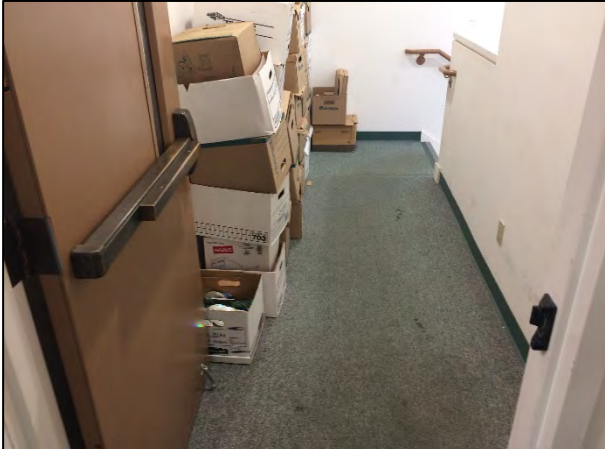
Boxes stored in exit stair
