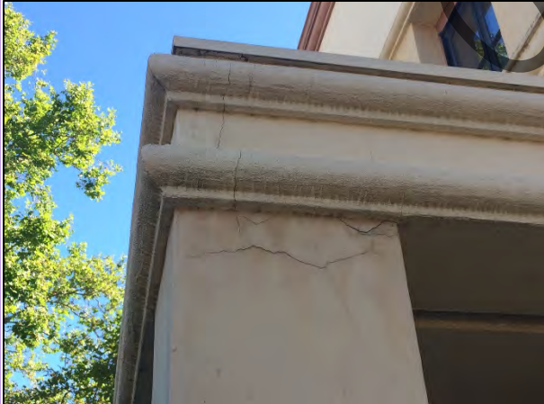
Stucco badly stained and cracked
