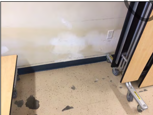
Wall and floor damage
