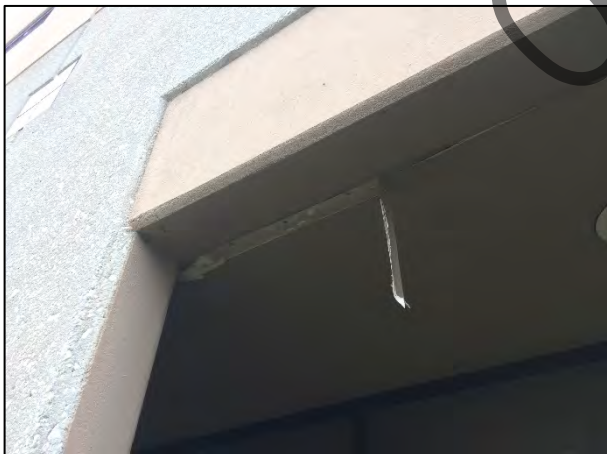
Failed GWB soffit
