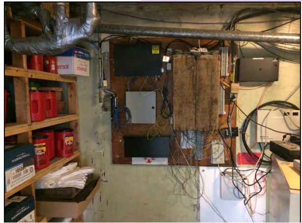
Utility Room, note wood box over equipment to prevent vermin chewing wires
