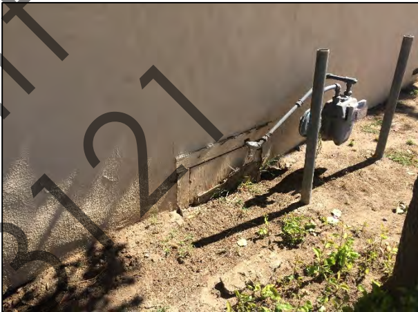
Gas meter at crawl space
