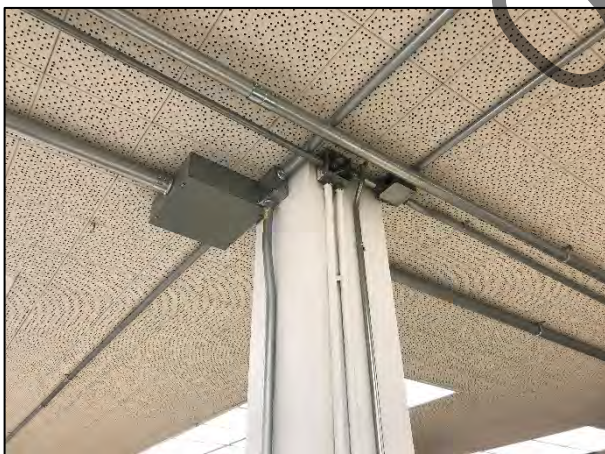
Exposed conduit in Reading Area
