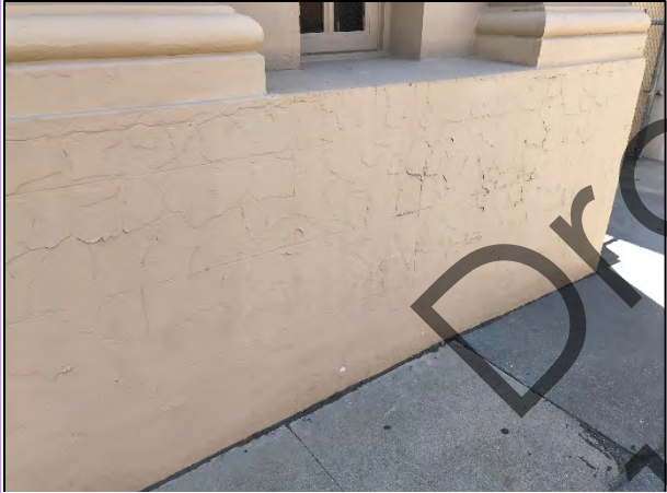
Peeling paint and stucco/plaster
