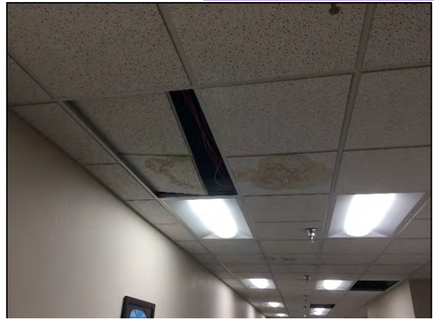
Stained ceiling tiles
