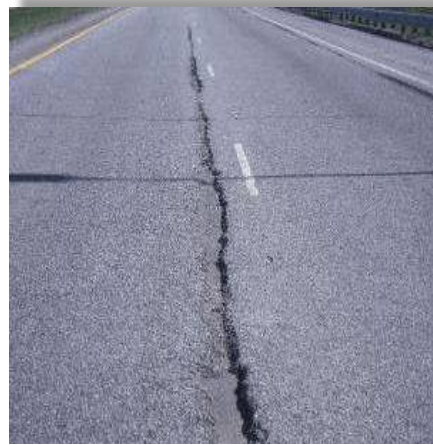
Transverse or Longitudinal Cracking
