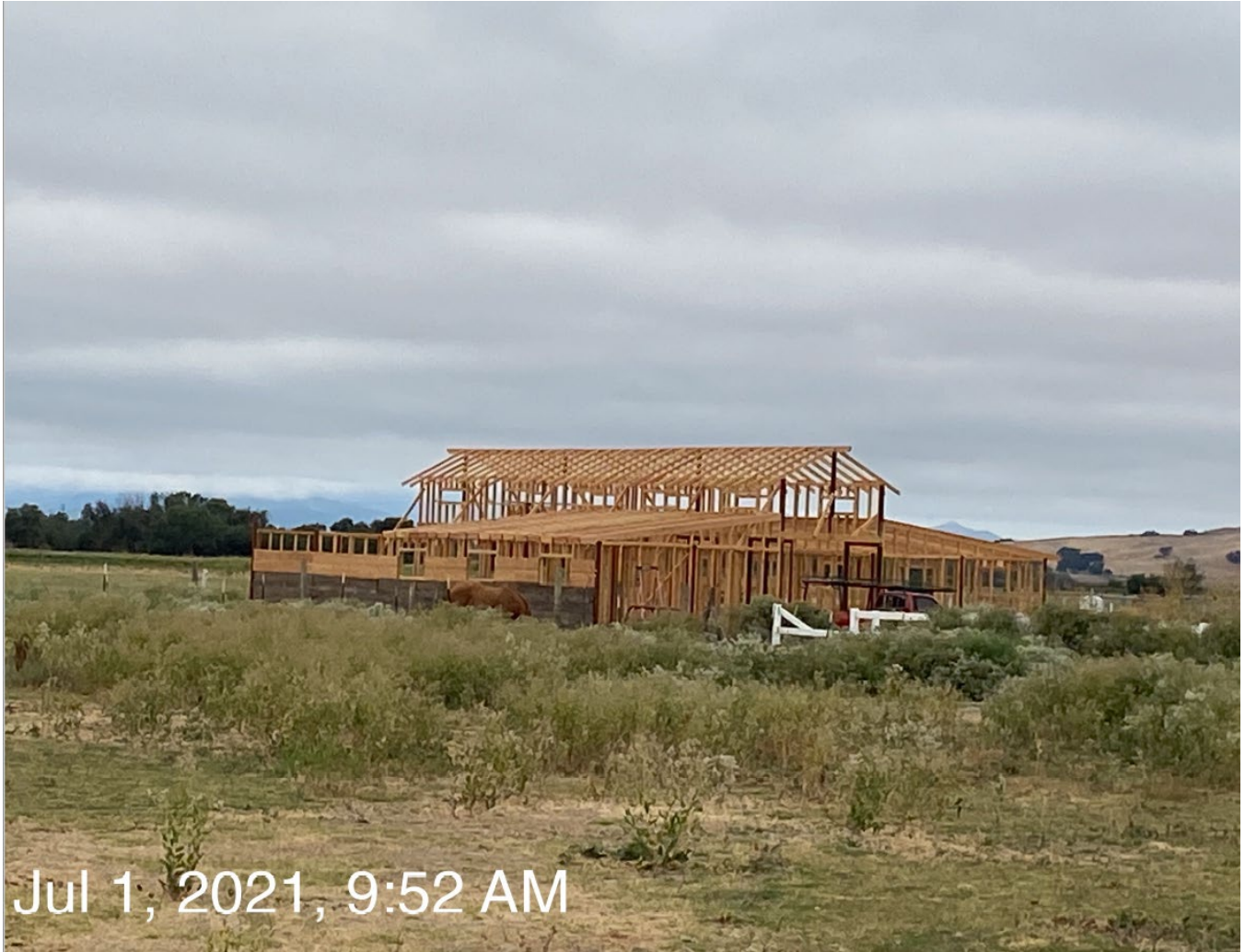
Exhibit C: Photo of active code violation
