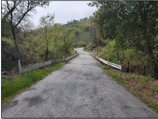
Existing Panoche Road Bridge looking northwest. 'S' curve in roadway would be eliminated.
