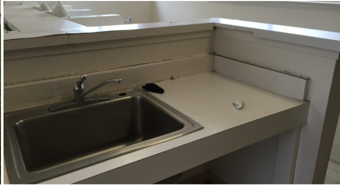
Laundry room wear and tear
