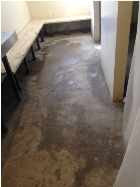
Poor drainage in shower area
